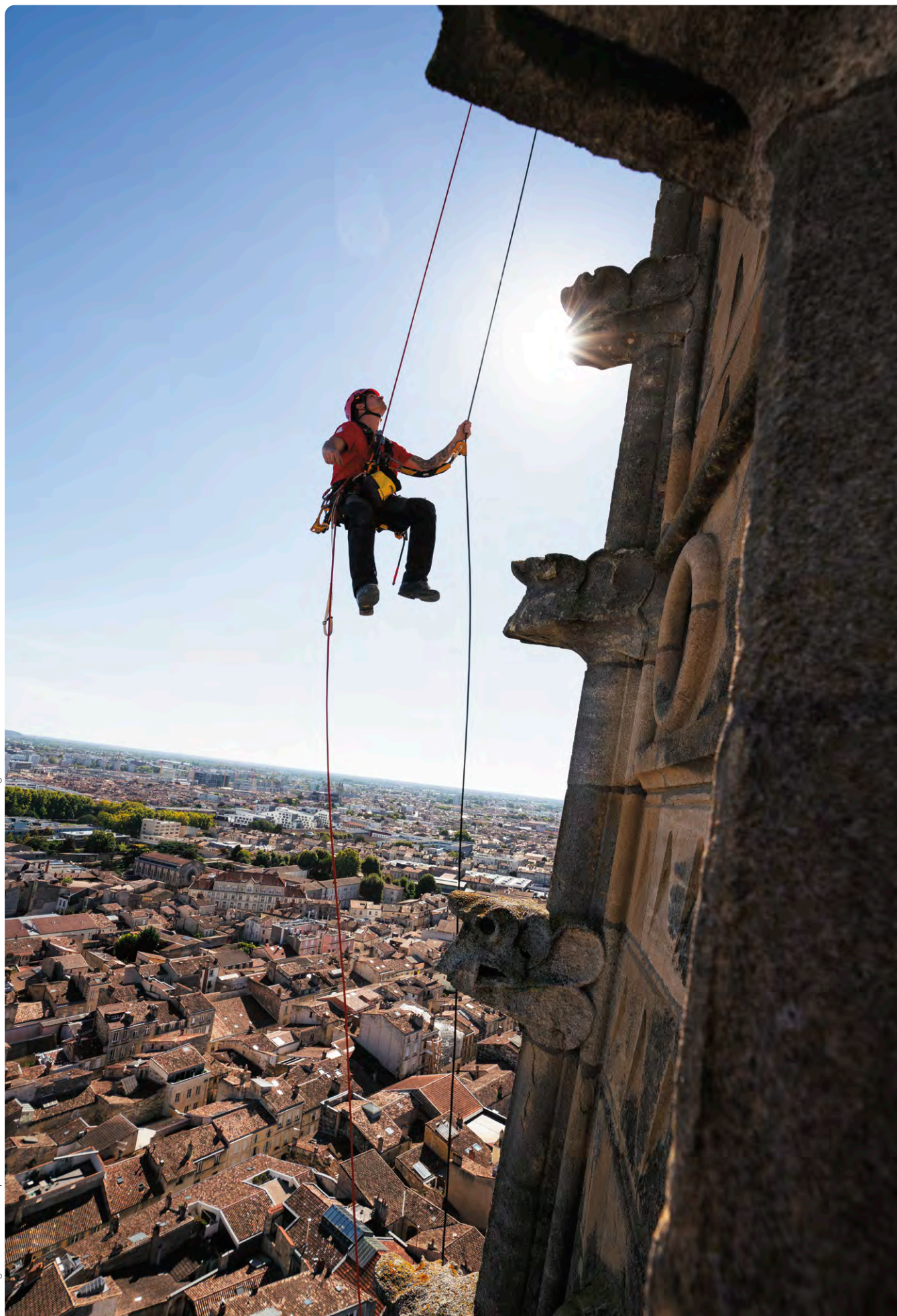
Installing monitors on the spire of the St Michel Church Bordeaux France © 2021 - Petzl Distribution - Vuedici.org - Adriénaline - Mairie de Bordeaux-DSC
